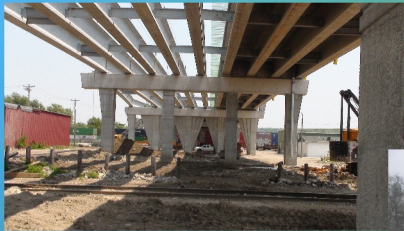
Broadway Viaduct, CB, IA 1537' x 60' Prestressed Bob, Ben, Doug, and Nels are working on the second stage. The traffic is traveling on the right hand side of the bridge.
