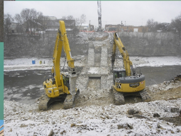
Iowa Falls, IA 289' x 42' Steel Arch Bridge Larry, Scott C, and Chad have almost finished the conc work and will be ready for steel.
