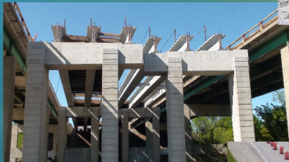
I-35 over EP True in WDM Dual 441' x 19' Prestressed Darren and Scott D are building these bridges in the median of the existing interstate.
