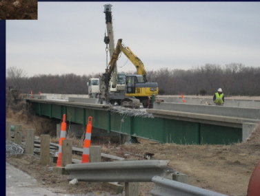
Harrison Co., IA Jeff and Brad are working on 2 Twin Overlays with Overhang Replacement
