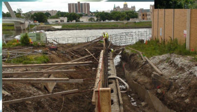
Corps Riverwalk Chuck and crew are building flood walls in downtown Des Moines.
