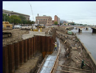
Corps Riverwalk Chuck and crew are building flood walls in downtown Des Moines.
