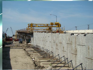
Broadway Viaduct, CB, IA 1537' x 60' Prestressed Bob, Ben and Doug are working to get the first half of this job poured before winter.
