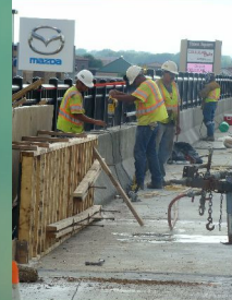
41st St Sioux Falls 305' x 112' Box Beam Neil's and Chad's crews poured it on at the end to earn the maximum incentive at Sioux Falls.
