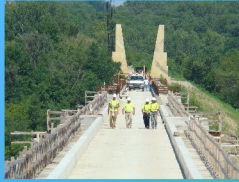
BOONE-DALLAS TRAIL BRIDGE 2530' X 12' TRAIL BRIDGE Scott C.'s crew finished up the bridge and the trail is being paved.
