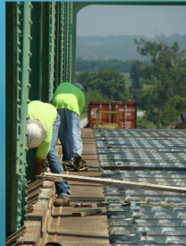
RTE 136 over MO River 1908' X 23' HIGH TRUSS Josh and Jake & company are replacing the deck here along with steel repairs.
