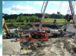
Saylorville Emergency Spillway 390' x 4' x 30' Trench Wall Larry has now poured over 3500 cy of concrete!
