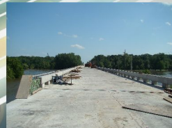
Mahaska Co., IA 1135' x 30' Steel Girder Evan's crew just finished this river bridge.
