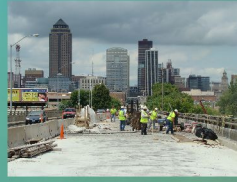
SW 7TH ST, DES MOINES 793' X 50' ARCH BRIDGE Tim's gang is overlaying this bridge, fixing joints and patching the arches.
